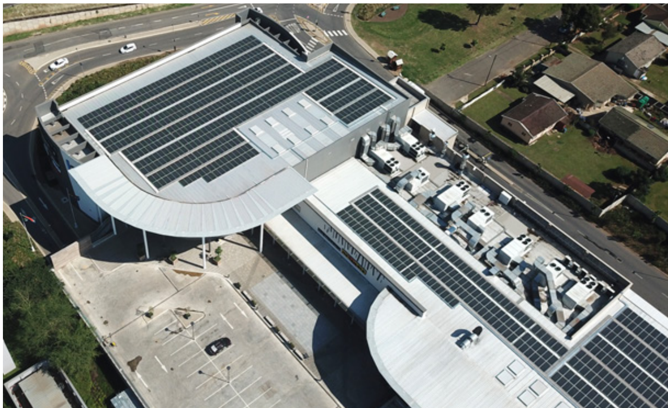
Rooftop solar PV array at Midlands Mall.
